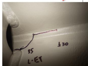
鋼床版のき裂
